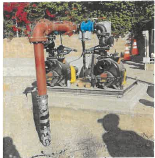
Piping previously installed to the duplex equalization pump.
