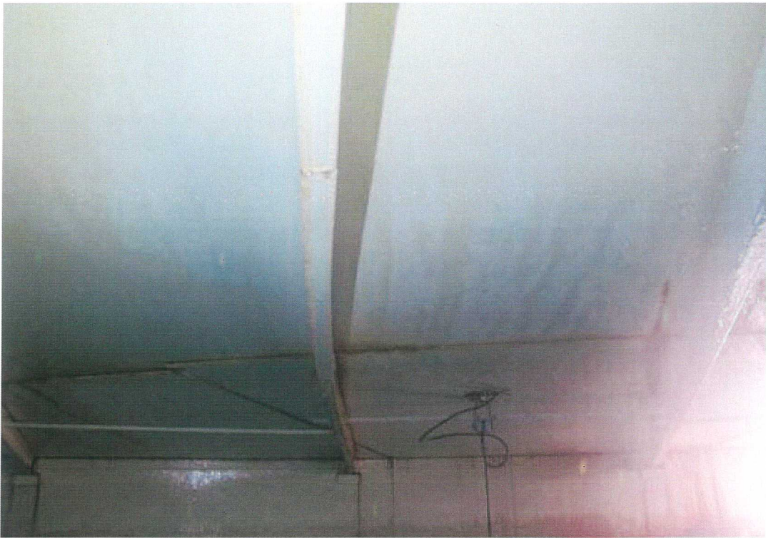
This photo shows an example of a bowed roof rafter.
