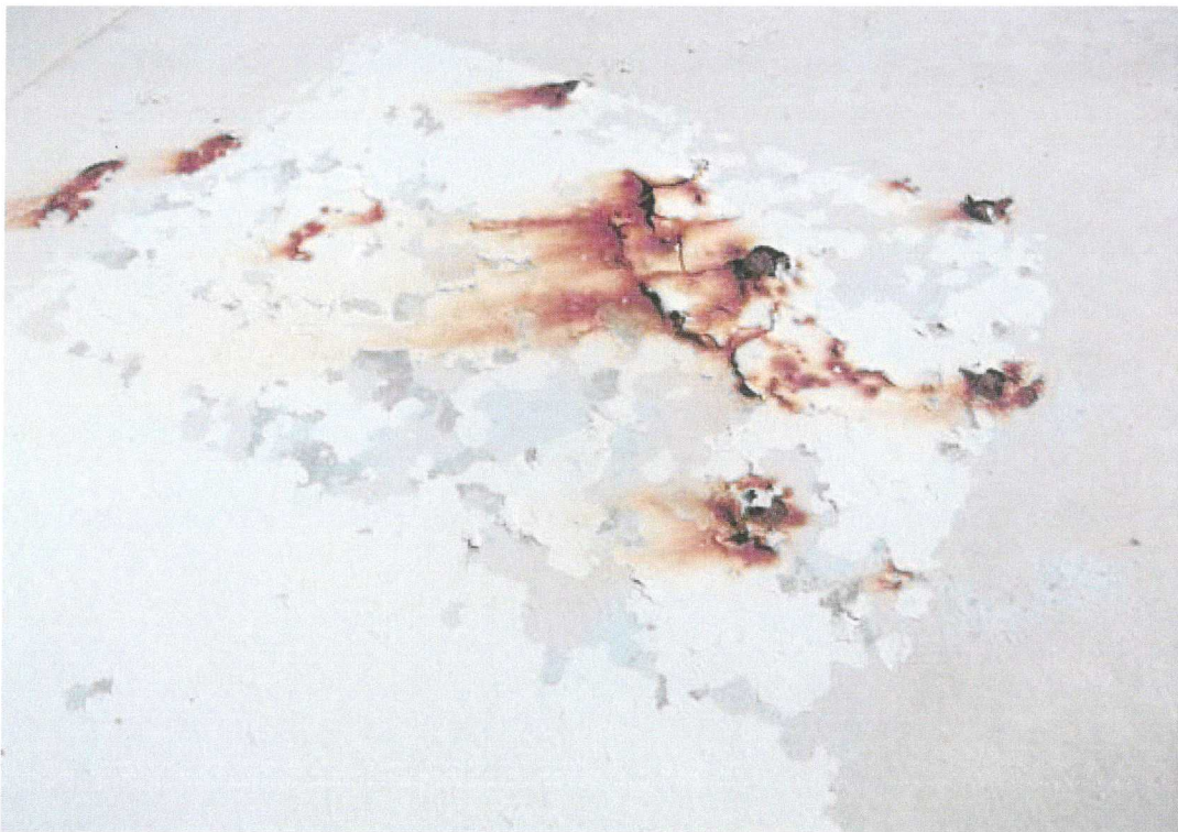
Another location of significant corrosion on the exterior roof. This location was spot repaired approximately 7 years ago.
