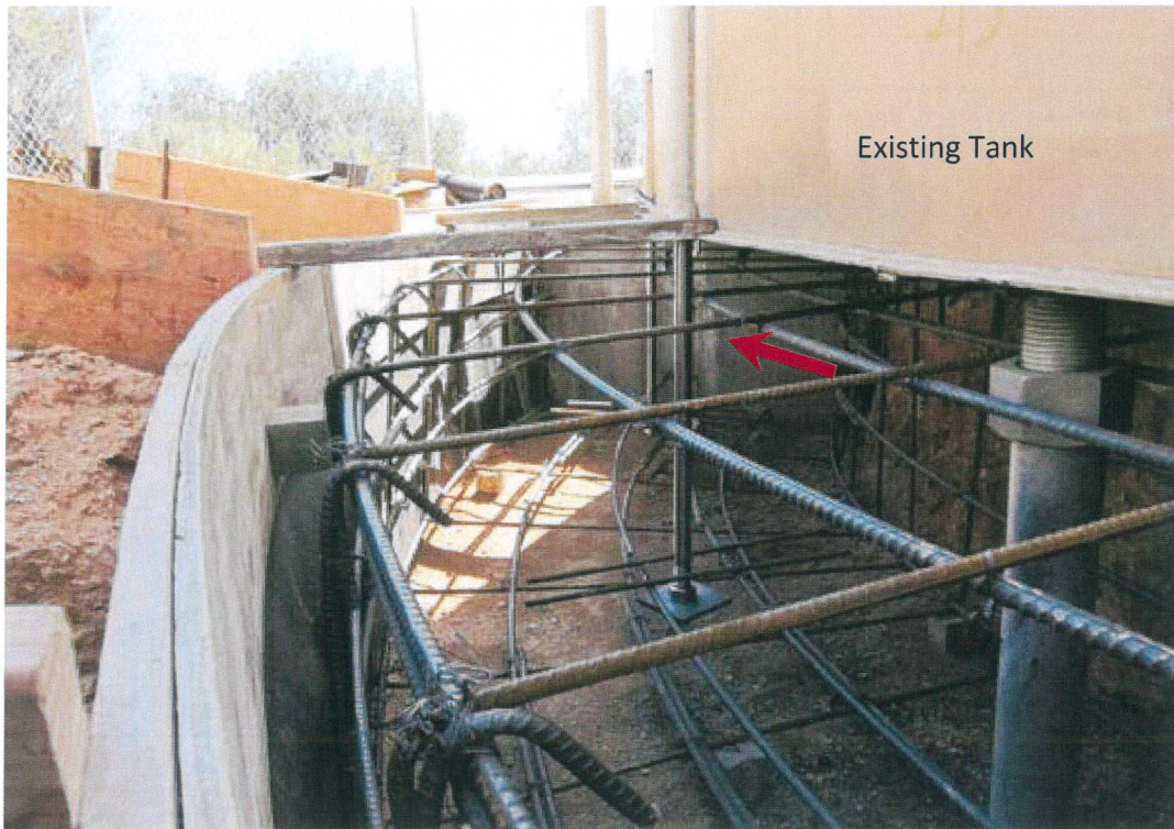
This photo shows the excavation, forms and rebar ready to place a concrete foundation under an existing tank. The arrow points to where concrete has already been installed as a part of this work.
