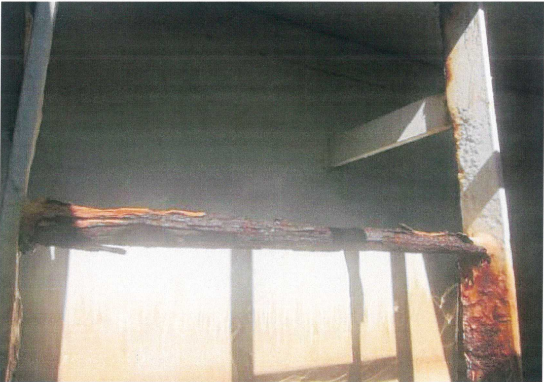
One of the severely corroded rungs on the interior ladder is shown above.
