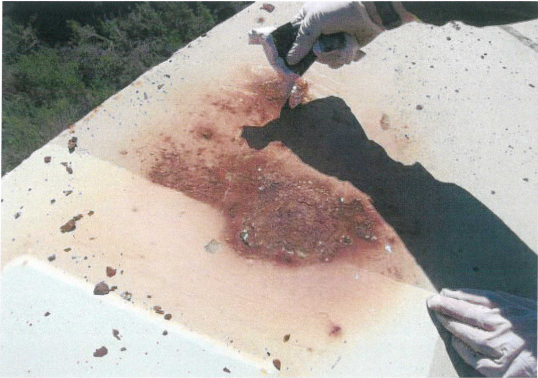
Significant corrosion on the exterior roof.
